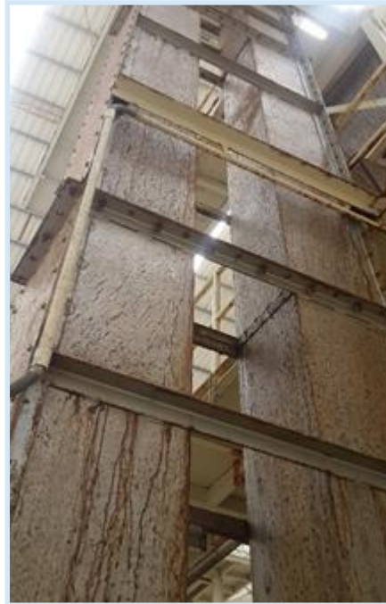
Closed system - cannot be cleaned
