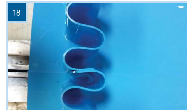
Sidewall Ready to be Re-welded Cut any excess strip from the sidewalls (Figure 17 & 18).
